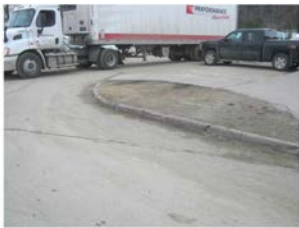
MHS-C9 Deteriorated asphalt curb
