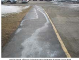
MVE-C4 Lack of Cross-Slope Resulting in Water Running Down Walk
