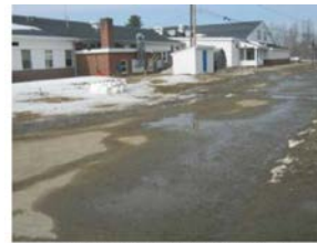
RES-C4 Puddles and deteriorated pavement at rear of building.
