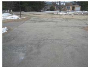
RES-C3 Deteriorated Sidewalk.
