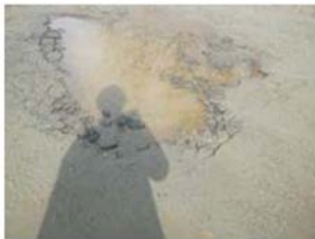
RES-C3 Pothole at side parking area.
