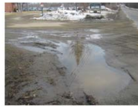
MVE-C3 Pothole at End of Bus Loop
