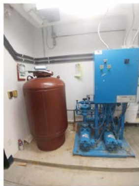
MMS-M1 Domestic Water Booster Pump System
