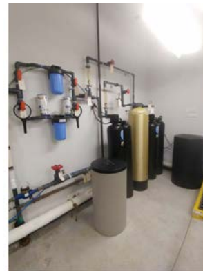
MMS-M2 Water Treatment System
